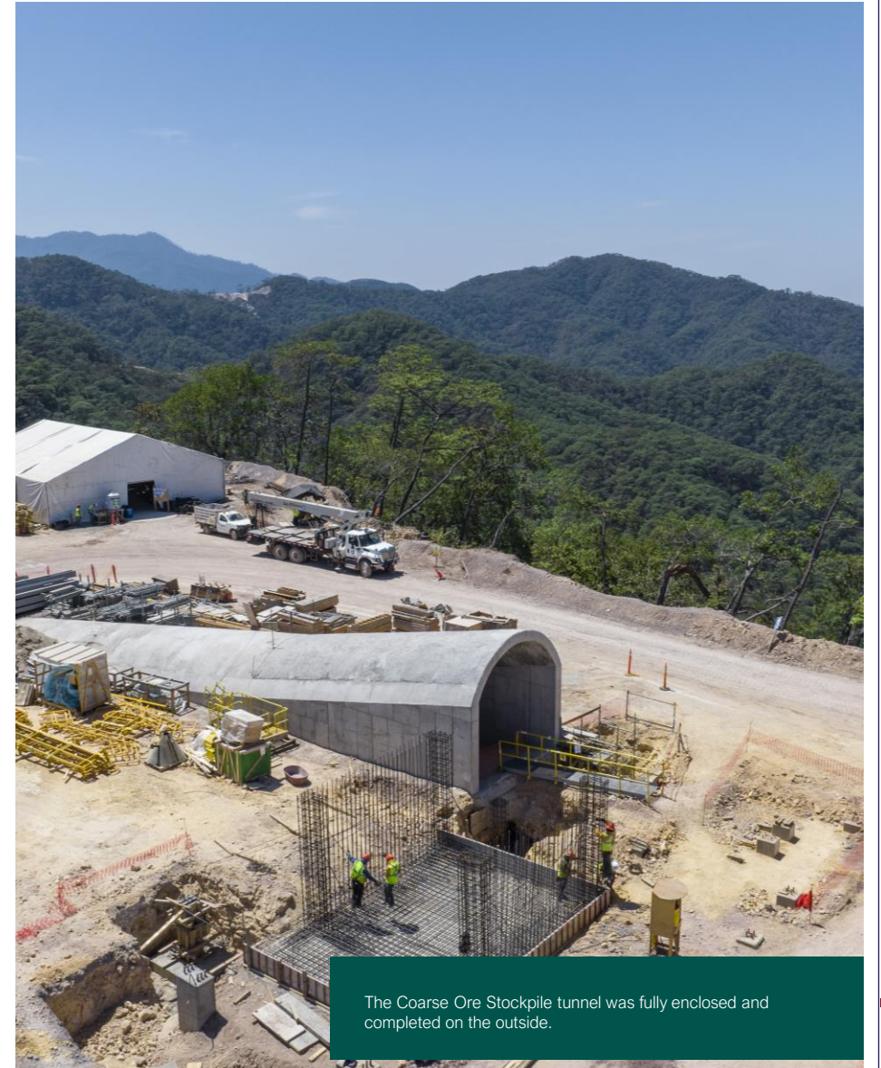
Excavation continues in the TSF embankment area and Lower Platform to allow for concrete work to start in Q2.
